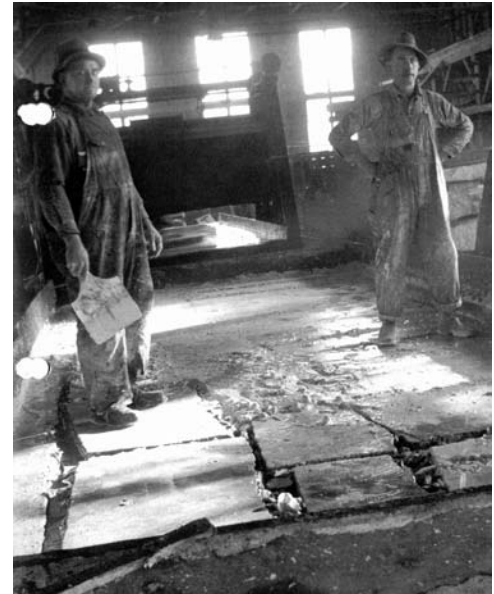
Figure 32 (above). Two bed setters in overalls filling the cracks between set stones with plaster. Note the bed setter on the left holding a wooden plaster paddle.
