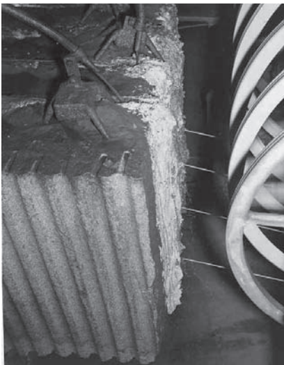
Figure 9 (left, top). A wire saw with four wires almost finished with the cut. Note the five sheaves, four of which are currently in use. Also, note the hoses conveying abrasive slurry into the saw kerfs. Figure 10 (left, bottom). Two- and three-strand saw wire.
